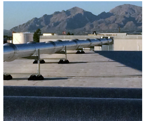
A pipe connecting several chilled-water systems was the solution to saving energy and money at our Tucson data center.
